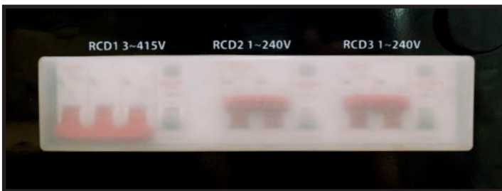
RCD protection for all high voltage circuits
